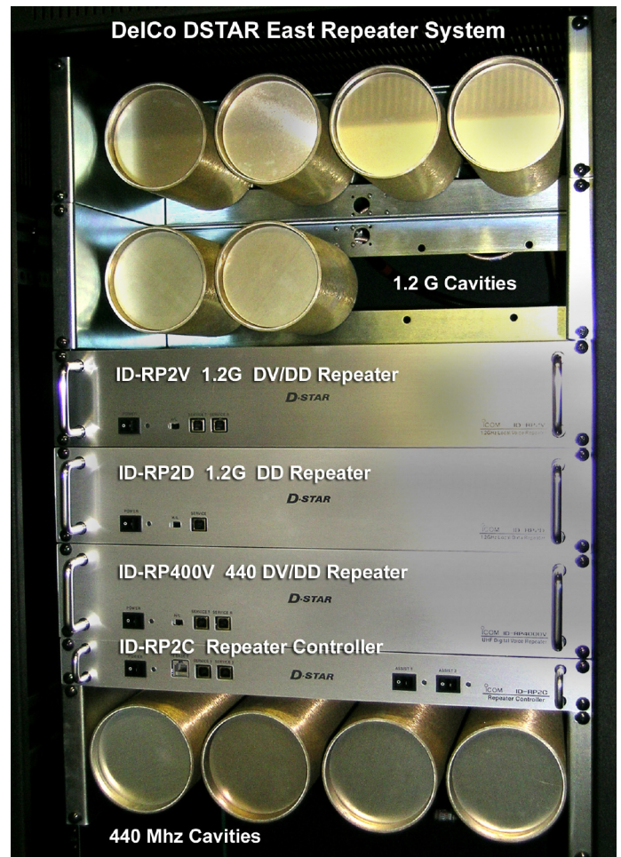
DELCO D-STAR EAST repeater system showing cavities, 440 DV repeater, 1.2G DV repeater, 1.2G DD repeater and controller
